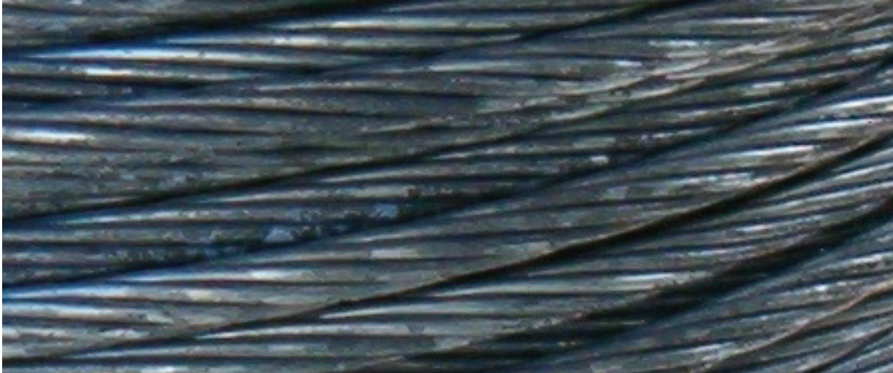
Figure 16. Oxidation on a conductor.
